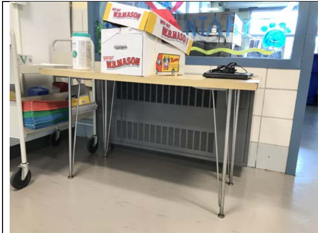
Unit Ventilator in School Entrance
