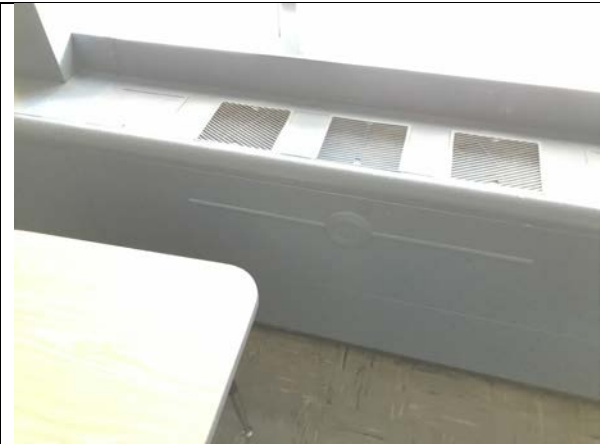
Unit Ventilator in Classroom
