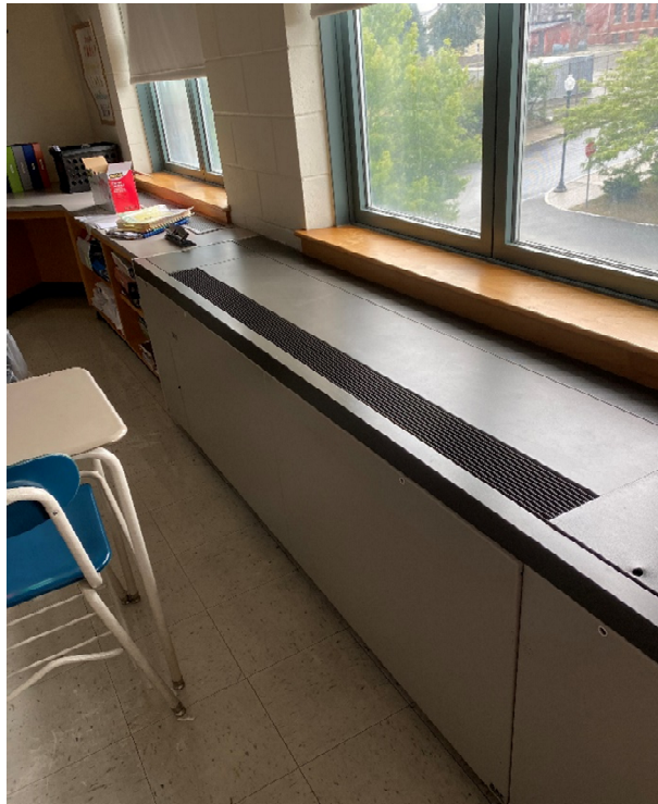
Picture #1: Typical Classroom Unit Ventilator (Sill Mounted)
