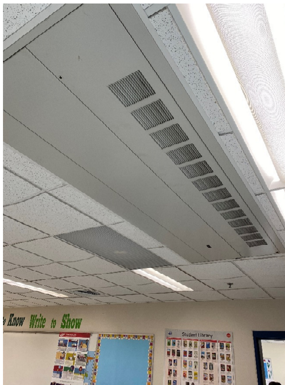
Picture #2: Typical Classroom Unit Ventilator (Ceiling Recessed)
