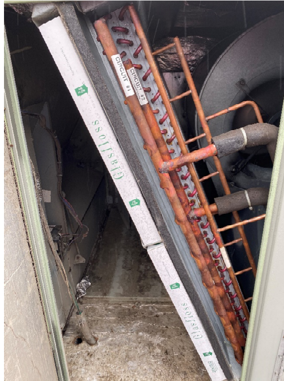
Picture #2: Typical RTU filtration
