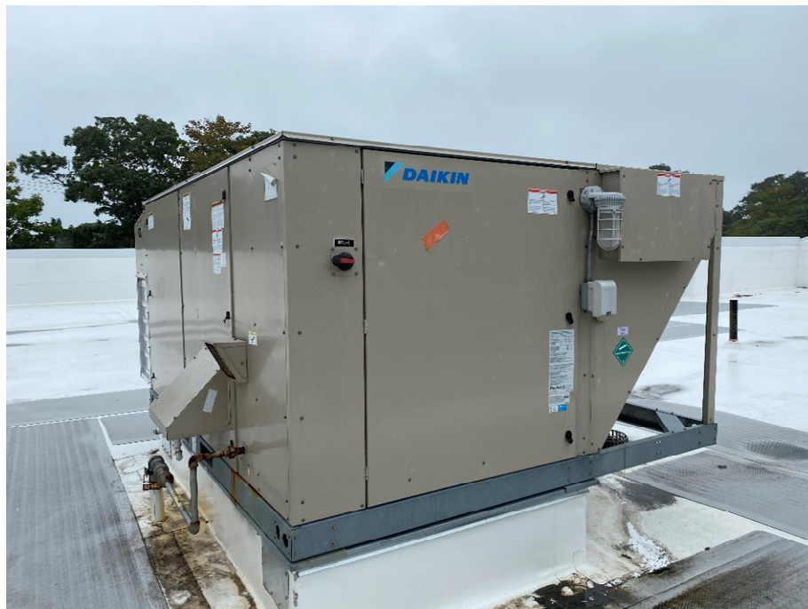
Picture #3: Typical Rooftop Unit (RTU)
