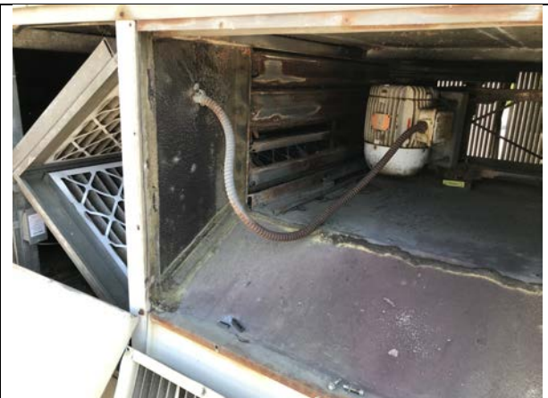
RTU Filter and Internals
