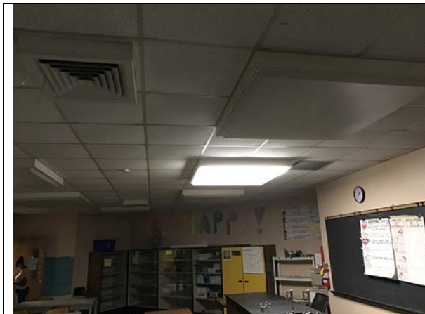
Classroom Supply Diffusers
