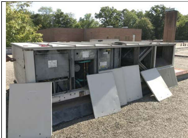
Roof Mounted Heating and Ventilating Unit (RTU)
