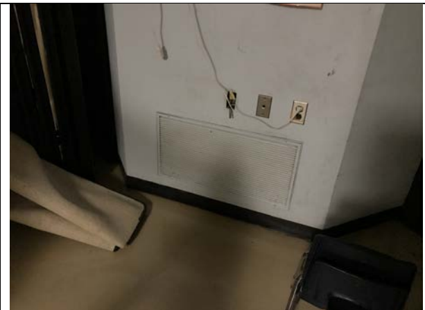
Classroom Return Grille
