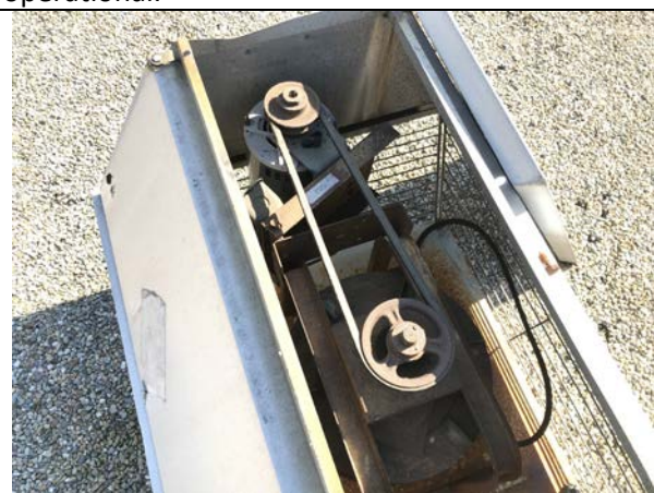
Typical Exhaust Fan (2)
