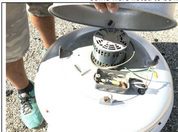
Typical Exhaust Fan (1)
