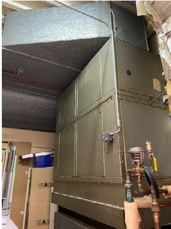
Picture #5: Auditorium / Café Heating Ventilating Unit
