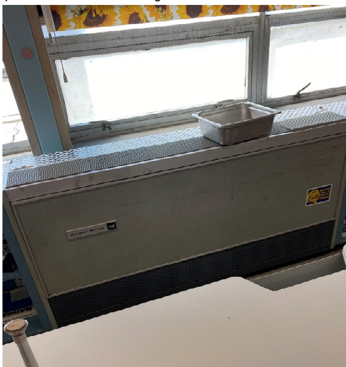
Picture #14: Typical Classroom Unit Ventilator
