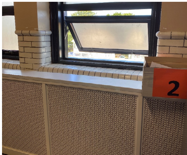
Picture #10: Typical Corridor Steam Radiator (with safety cabinet)
