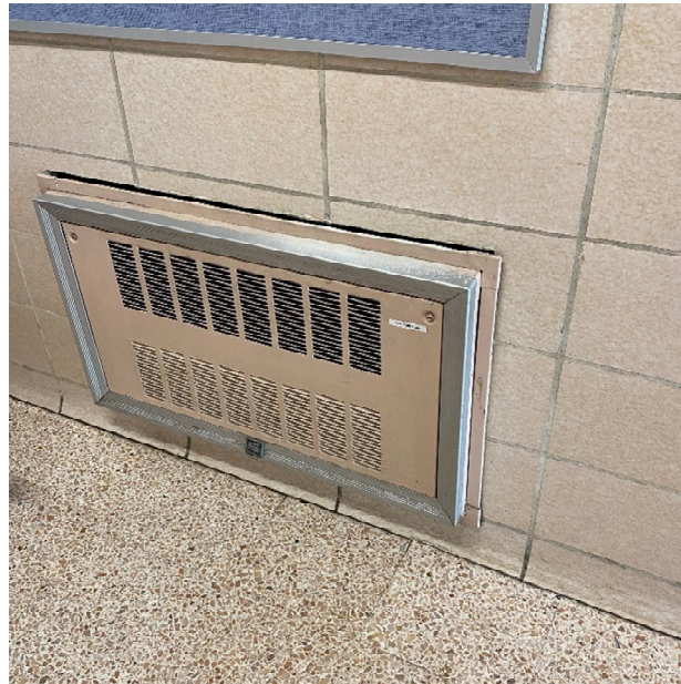
Picture #2: Typical Corridor Cabinet Heater
