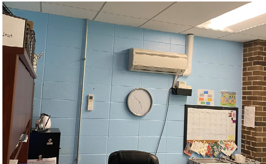
Picture #6: Administration Office / DX Fan Coil
