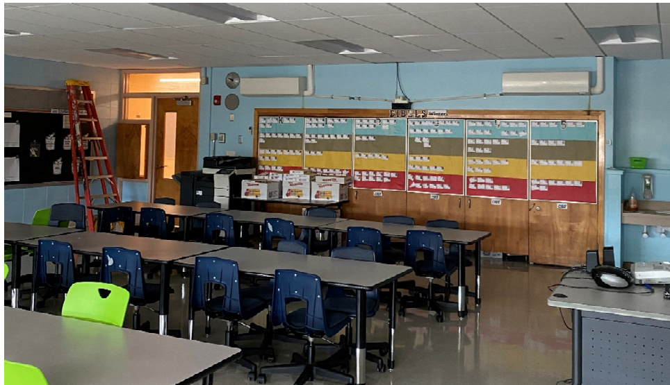
Picture #7: Miscellaneous Classroom / DX Fan Coil
