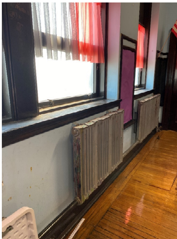
Picture #8: Typical Classroom Steam Radiator and Operable Windows
