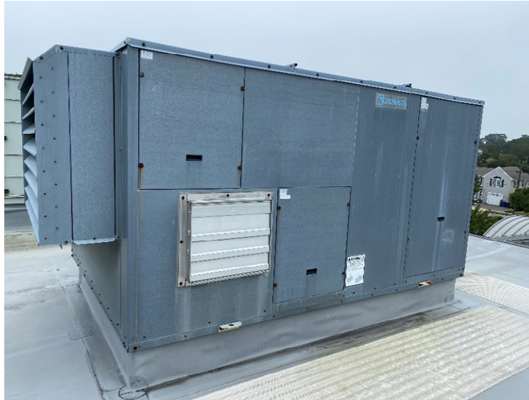
Picture #6: Typical Energy Recovery Unit
