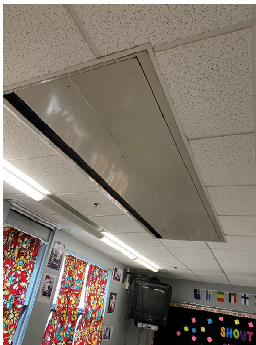
Picture #2: Typical Classroom with ceiling recessed Unit Vent
