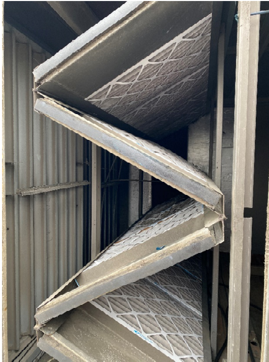
Picture #4: Typical RTU filtration
