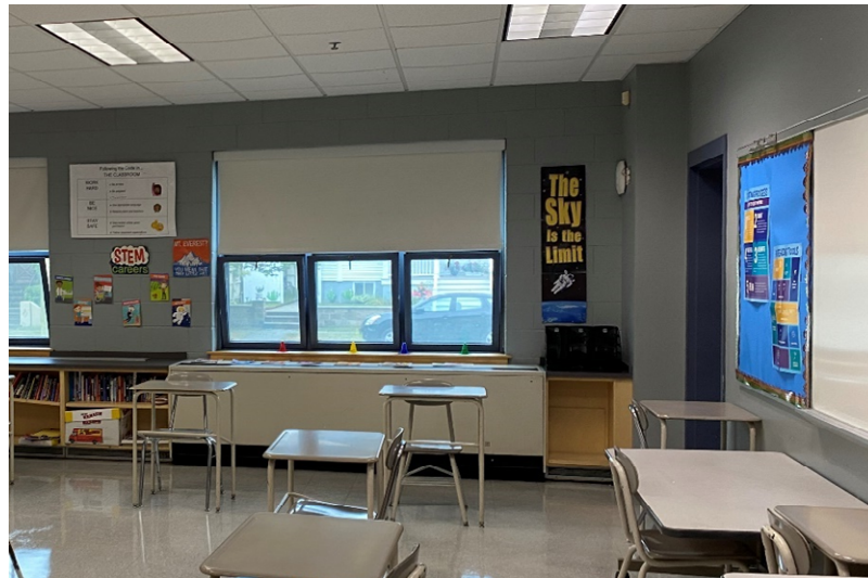
Picture #1: Typical Classroom with sill mounted Unit Vent
