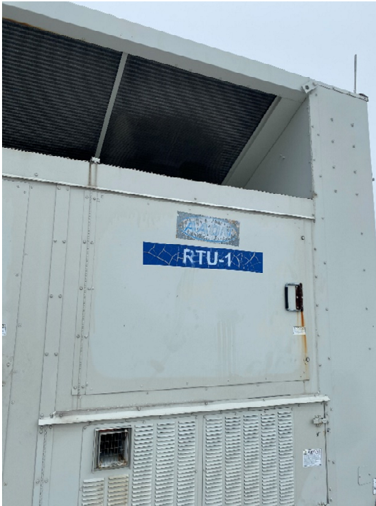
Picture #1: Typical Rooftop Unit
