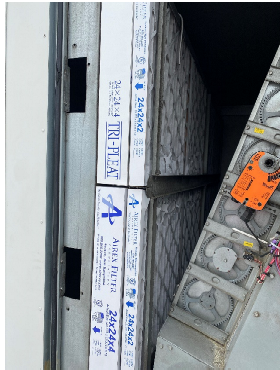
Picture #2: Rooftop Unit Supply air Filtration
