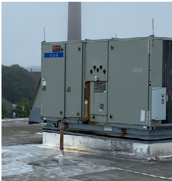
Picture #3: Rooftop Unit 6
