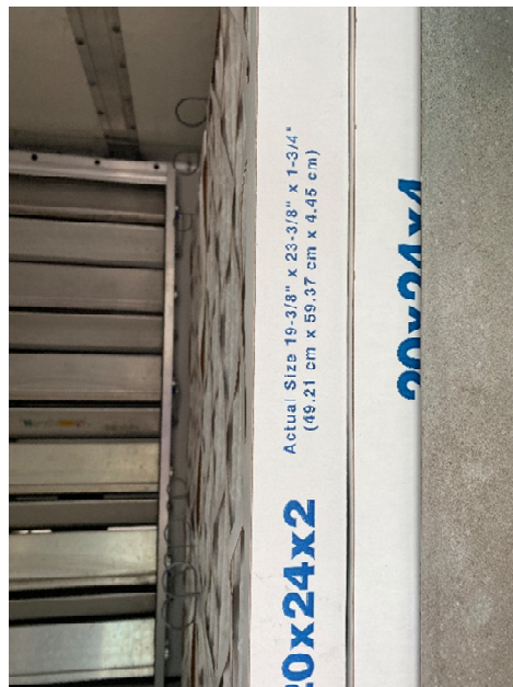
Picture #3: Pre and Final filter within Café / Audi Rooftop Unit
