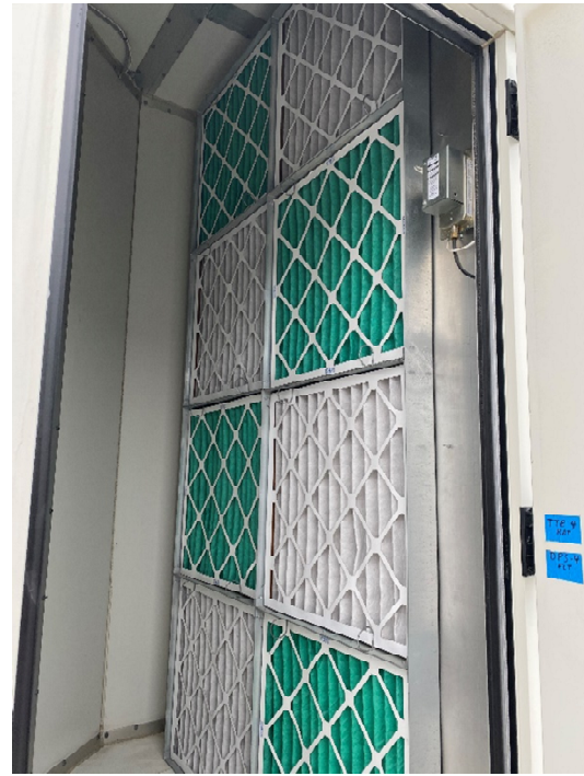
Picture #2: Rooftop Unit MERV-7 Filters
