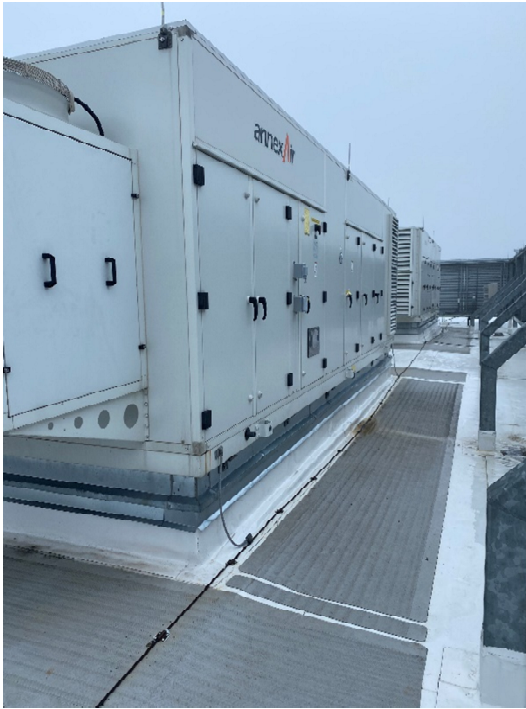
Picture #1: Typical Rooftop Unit
