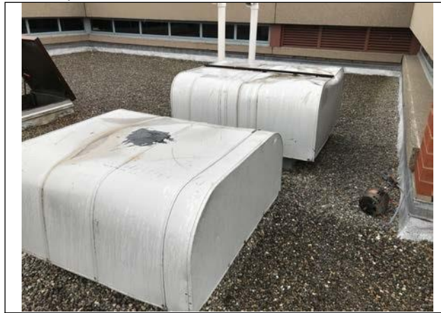
Typical Exhaust Fan (1)
