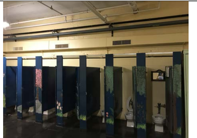
Girls Bathroom Exhaust Duct
