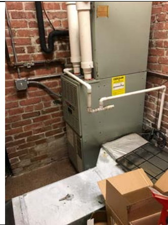
3 rd Floor Classroom HVAC Unit
