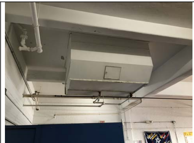
Cafeteria Heating Unit
