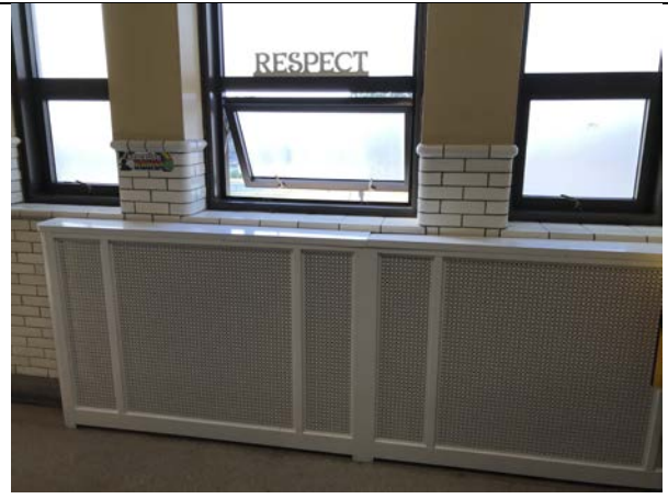
Typical Hallway radiation
