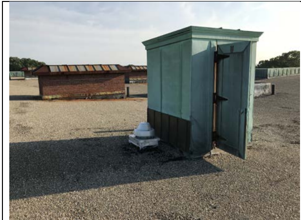
Teachers Bathroom Exhaust Fan
